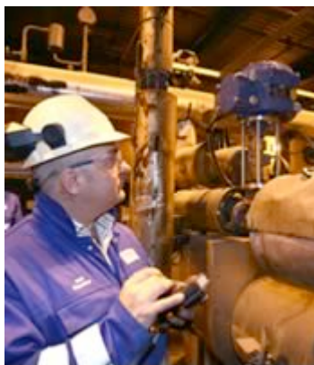
Rotork CVA actuator installation at a UK power station.
